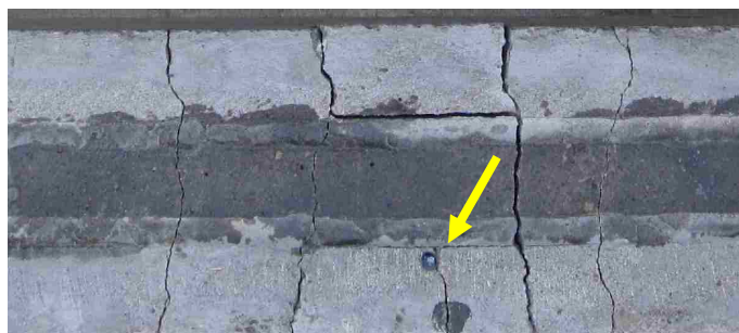
Figure 5.20. Close-up view of the crack pattern within the midspan of the tension face of the Beam # 6
