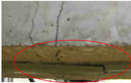
Figure 5.10. Crack pattern difference between Beam # 3 and Sensor # 3 and delamination of HoldTight 102 adhesives at midspan
