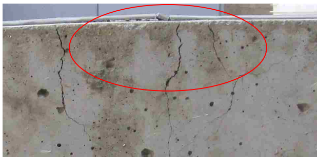
Figure 5.7 HoldTight 102 spalling at the midspan of Beam # 2
